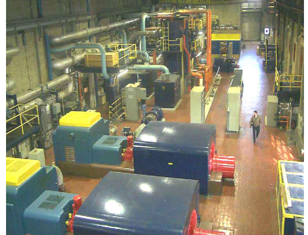
University of Michigan Turbine Room
