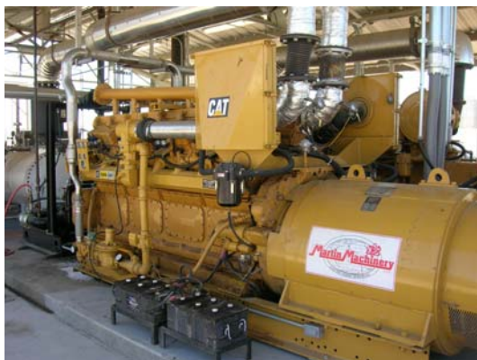
Picture above: 400 kW reciprocating engine
