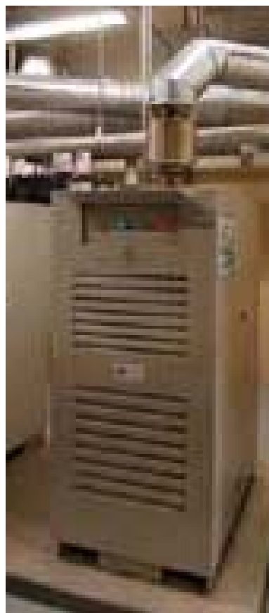
30 kW Capstone Microturbine at the Albert Lea Wastewater Treatment Facility
