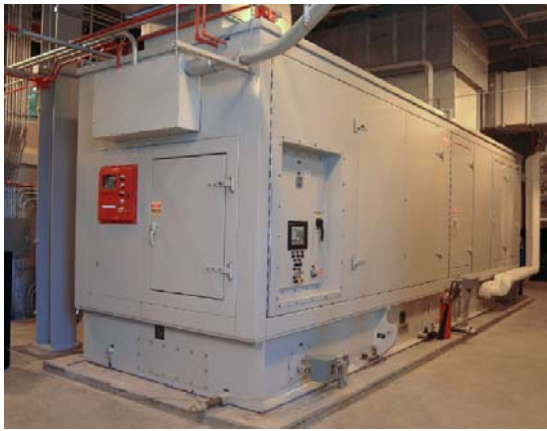
5.5 MW Solar Taurus 60 Turbine Generator
