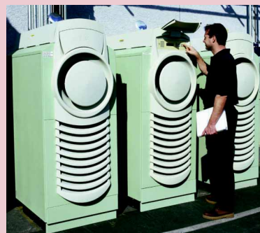
Multiple microturbine installation.
