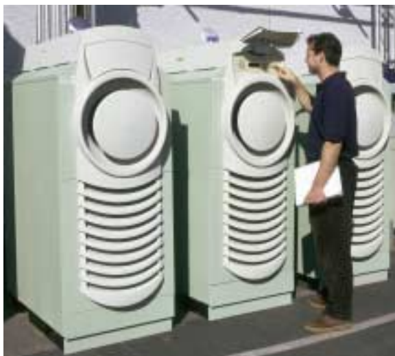
Figure 15: Microturbine Installation (Photo Courtesy of Capstone Microturbine Corp.)
