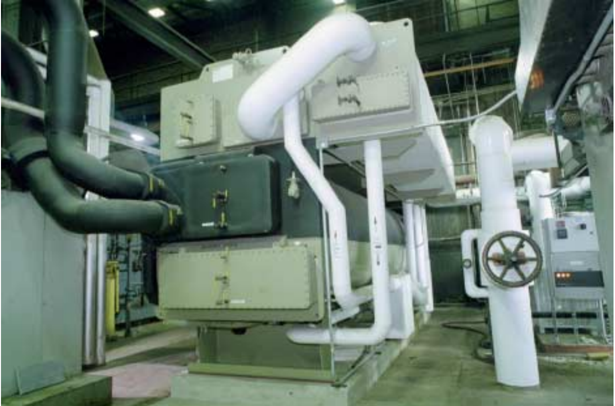
Figure 22: Large Absorption Operating on Waste Heat from Engine Generators Equipment Located at the University of Illinois at Chicago Power Plant (Photo Courtesy of the University of Illinois at Chicago.)
