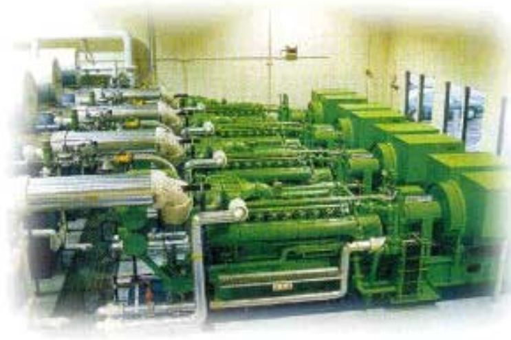
Figure 17: Engine Generating Plant
