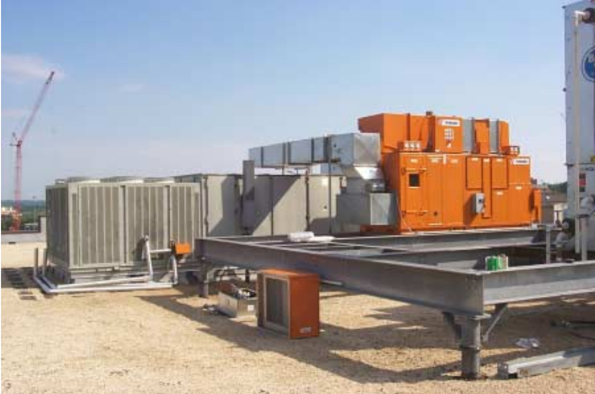
Figure 23: Desiccant Dehumidifier Operating at the University of Maryland (Photo Courtesy of the Department of Energy)
