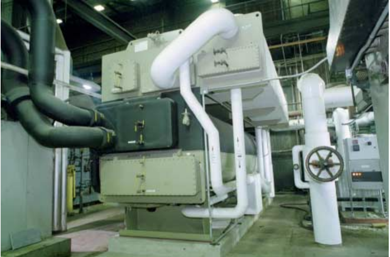
Figure 22: Large Absorption Operating on Waste Heat from Engine Generators Equipment Located at the University of Illinois at Chicago Power Plant (Photo Courtesy of the University of Illinois at Chicago.)
