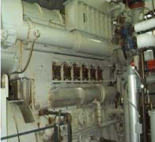
Figure 5: Fairbanks – Morse Generator Set
