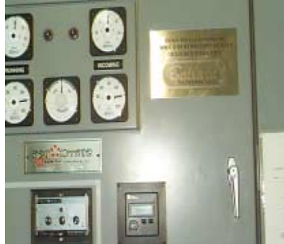
Figure 6: GE Zenith Energy Commander in the Control Room
