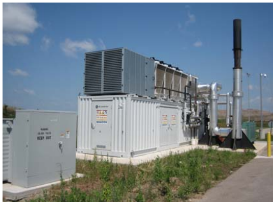
GE Jenbacher Container with Heat Recovery Equipment
