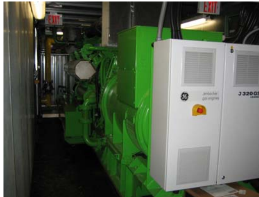
GE Jenbacher J320 Engine Generator
