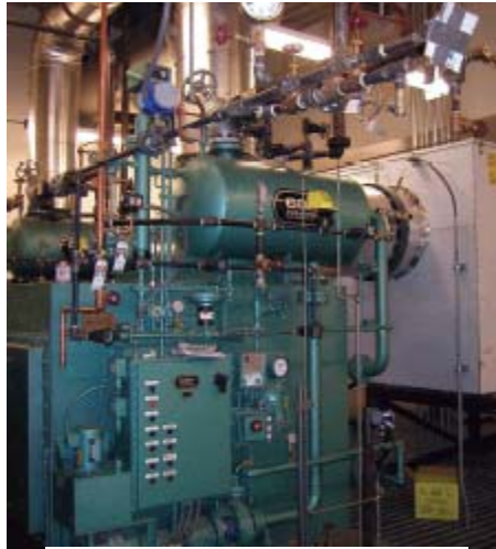
Heat recovery steam generator
