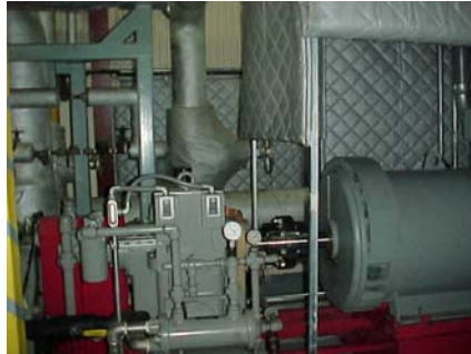
600 kW turbine installed in 1999
