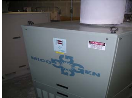
The MicoGen heat recovery system
