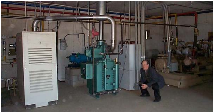
The CHP system at Colorado Pork: Capstone microturbine (far left), Caterpillar engine (far right) and balance of plant
