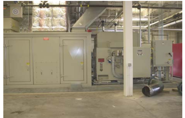
Utah State University's 4.5-MW gas-fired turbine was installed as part of an expansion to the central utility plant.
