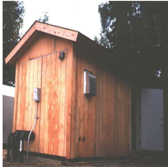
Figure 3: School Boiler Module
