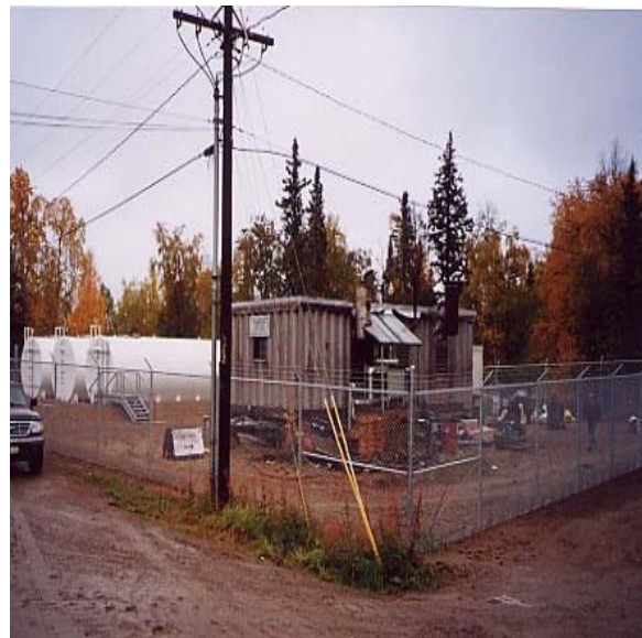
Figure 1: Anvik Power Plant
