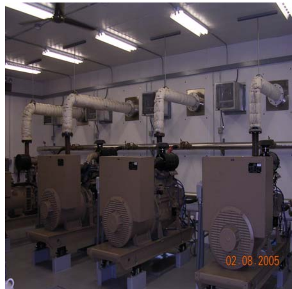
Figure 1: Golovin Power Plant
