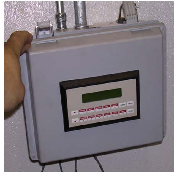
Figure 3: Energy Meter Display
