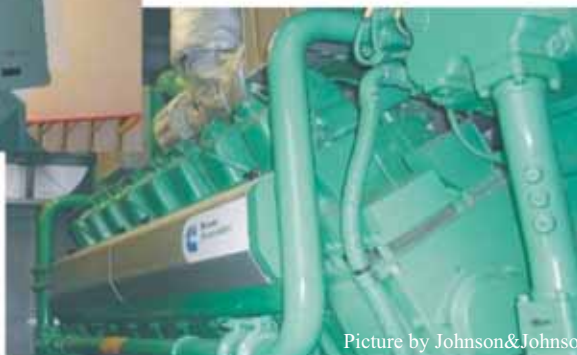
Picture below: 16-cylinder 1,100 kW reciprocating engine from Cummins.
