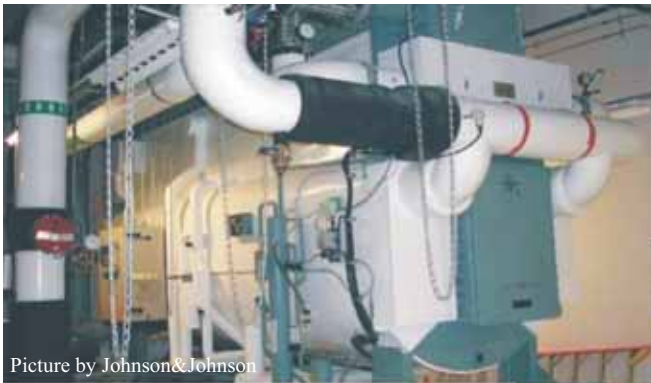
Left hand side: 500 RT (refrigeration ton) absorption chiller.
