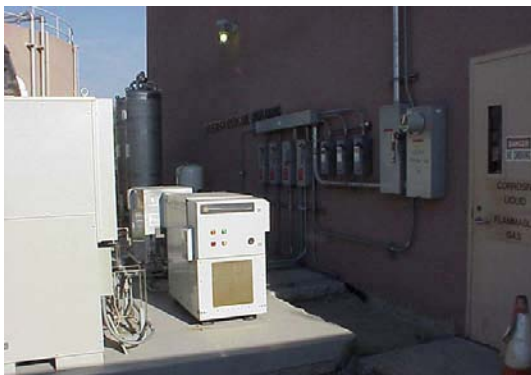
Picture above: Microturbine disconnection switches
