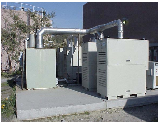
Picture below: Microturbines
