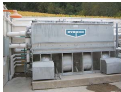
EvapCo cooling tower with electrostatic discharge
